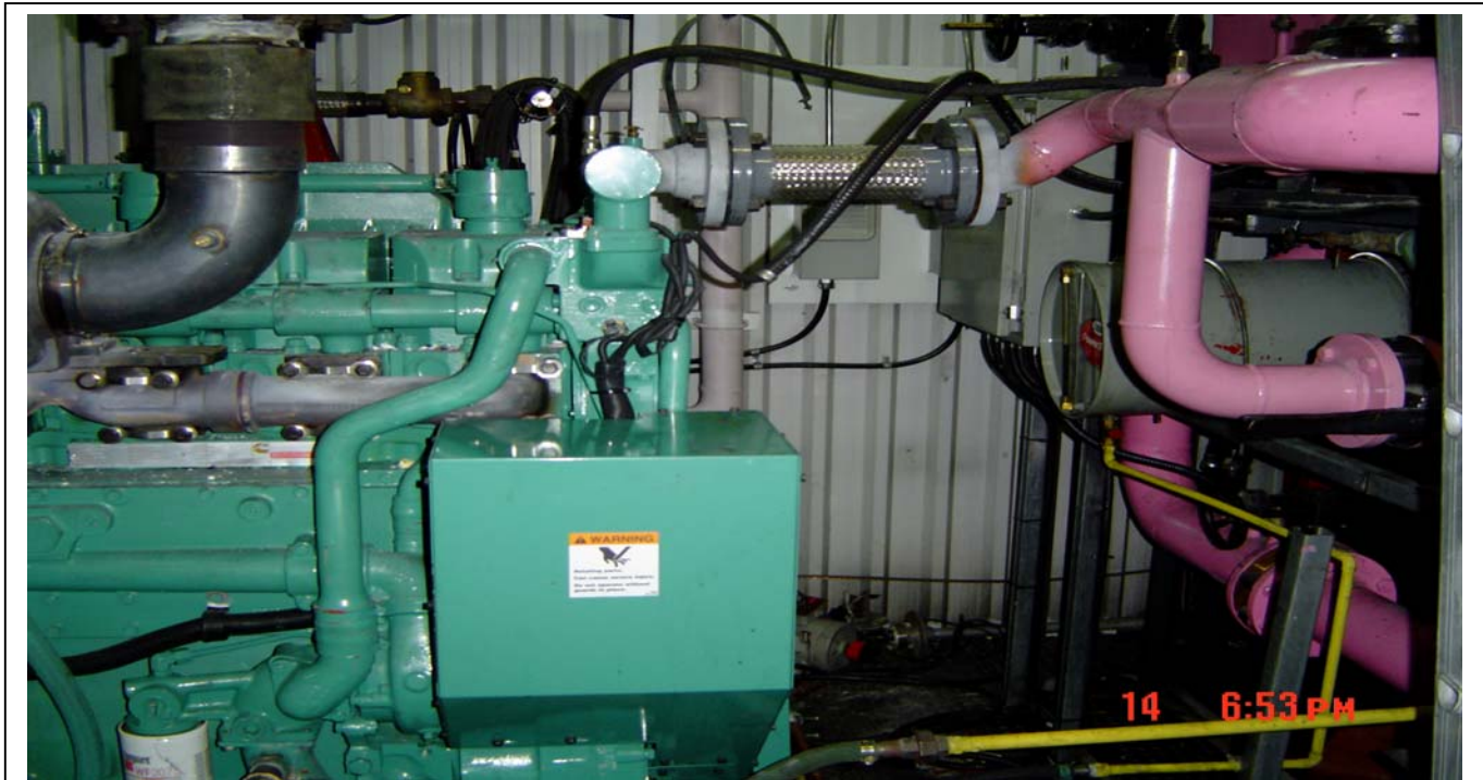
▼ Retrofitted Piping Connections
