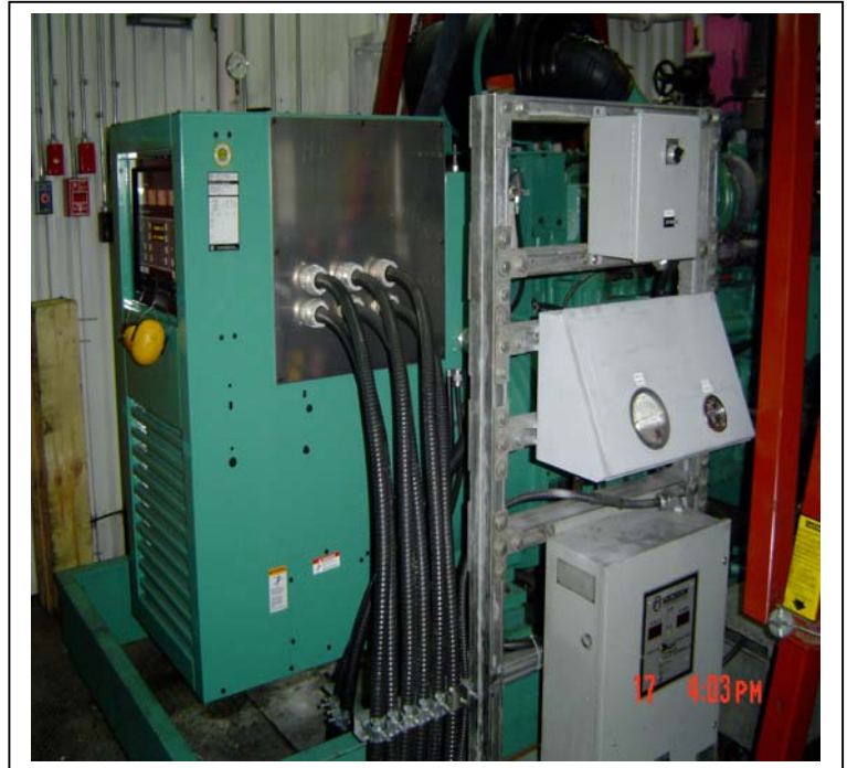
▲ Existing Power and Control Feeds (Reused)
